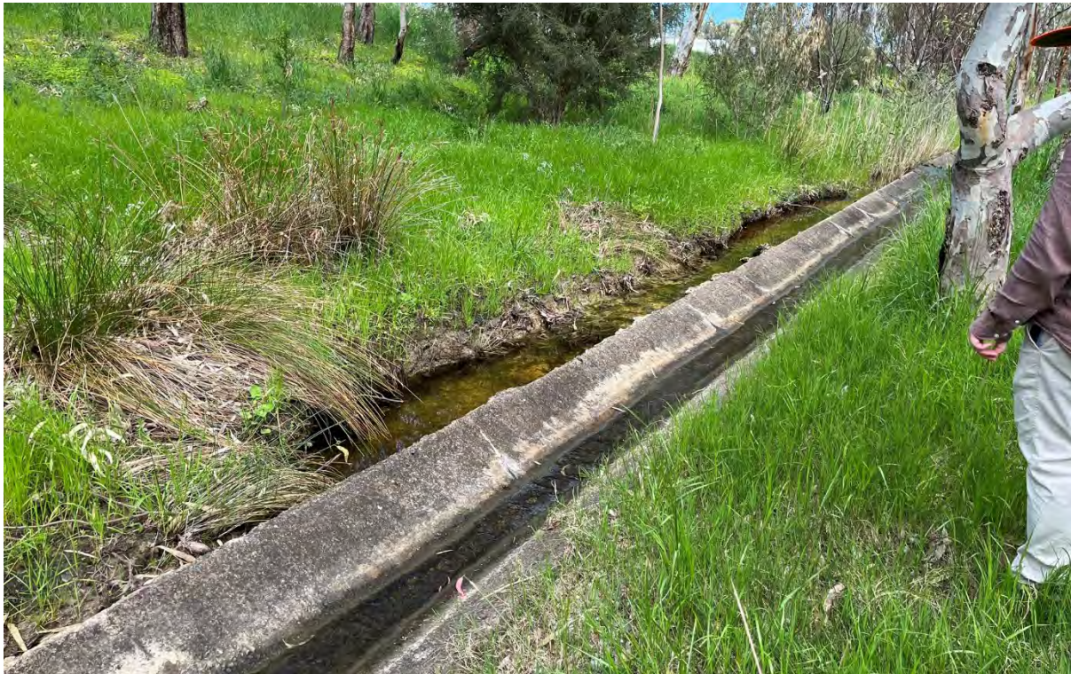
Figure 5 Reynella East College concrete lined channel (with erosion)
