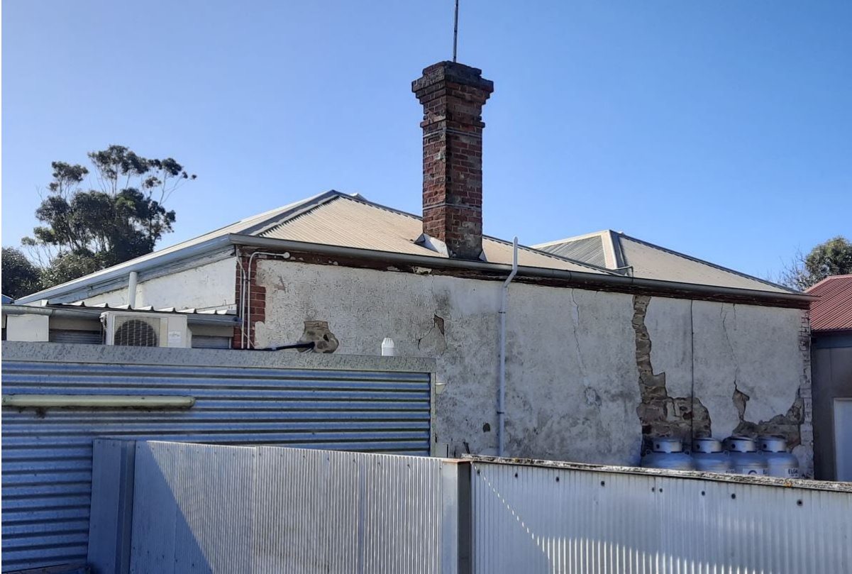
Minimal surviving heritage fabric at Victory Hotel, 652 Old Sellicks Hill Road, Sellicks Hill (GGA, 2021).
