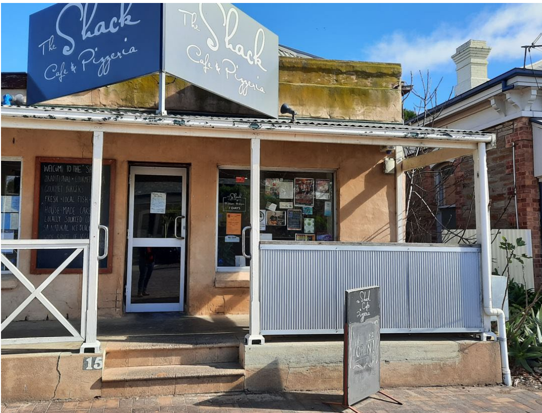
Deterioration to parapet wall with extensive modifications to original frontage (GGA, 2021).
