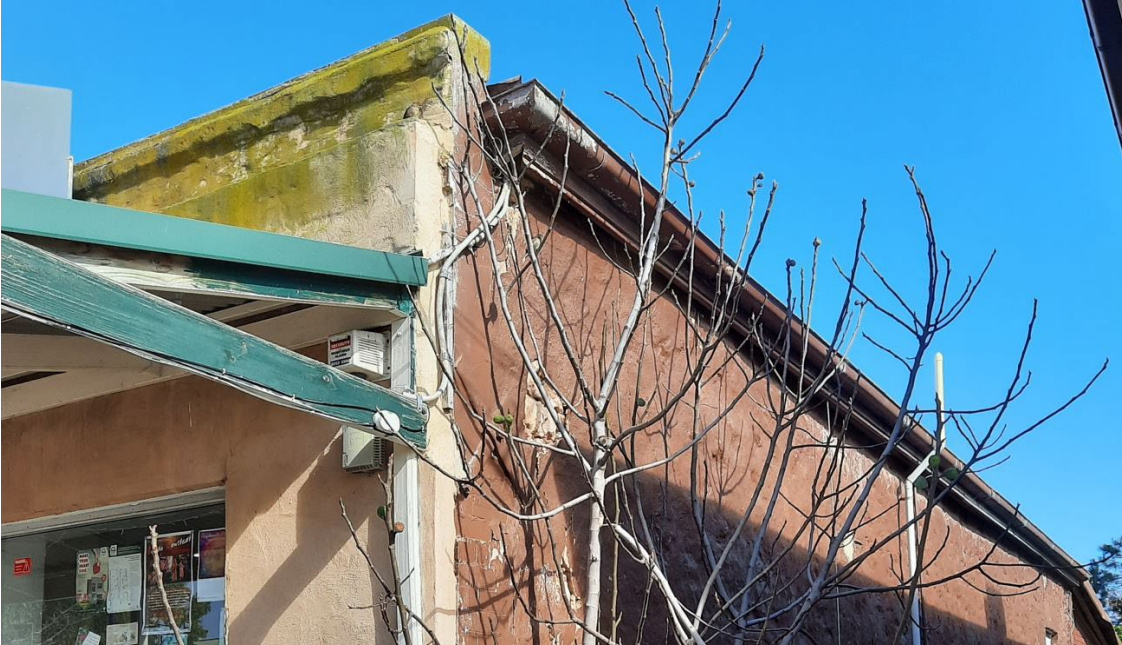
Deterioration to parapet wall with heritage fabric to north elevation (GGA, 2021).
