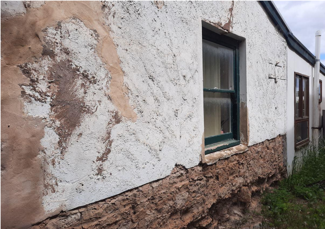
East elevation of former cottage, early masonry in poor condition at lower level with cement rendering from mid-level. Original iron wall plating at upper level. Late 20 th century additions about early lean-to additions to the immediate north (GGA, 2021).
