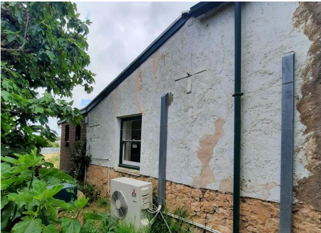
West elevation of former cottage, early masonry in poor condition at lower level with cement rendering from mid-level. Original iron wall plating at upper level. Mid-20 th century additions about early lean-to additions to the immediate north (GGA, 2021).
