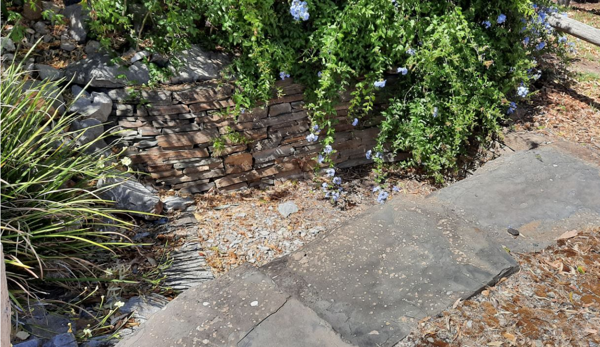
C.1864 dry stone walls and slate capping to culvert's southern end near 33 St Andrews Terrace; recent landscaping associated with 4 St Judes Street infringes the historic fabric (GGA, 2022).
