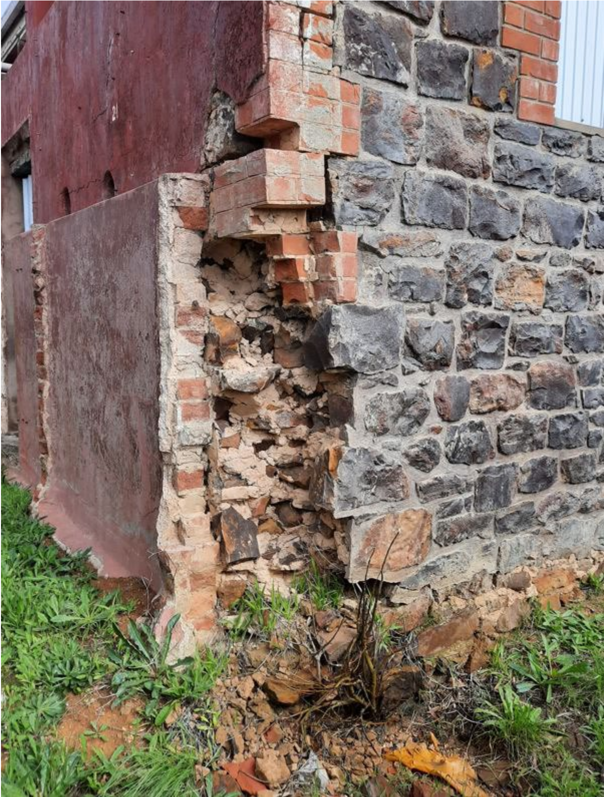
Deterioration of masonry fabric to north-east corner of building, presenting some hazard to adjoining properties (GGA, 2021).
