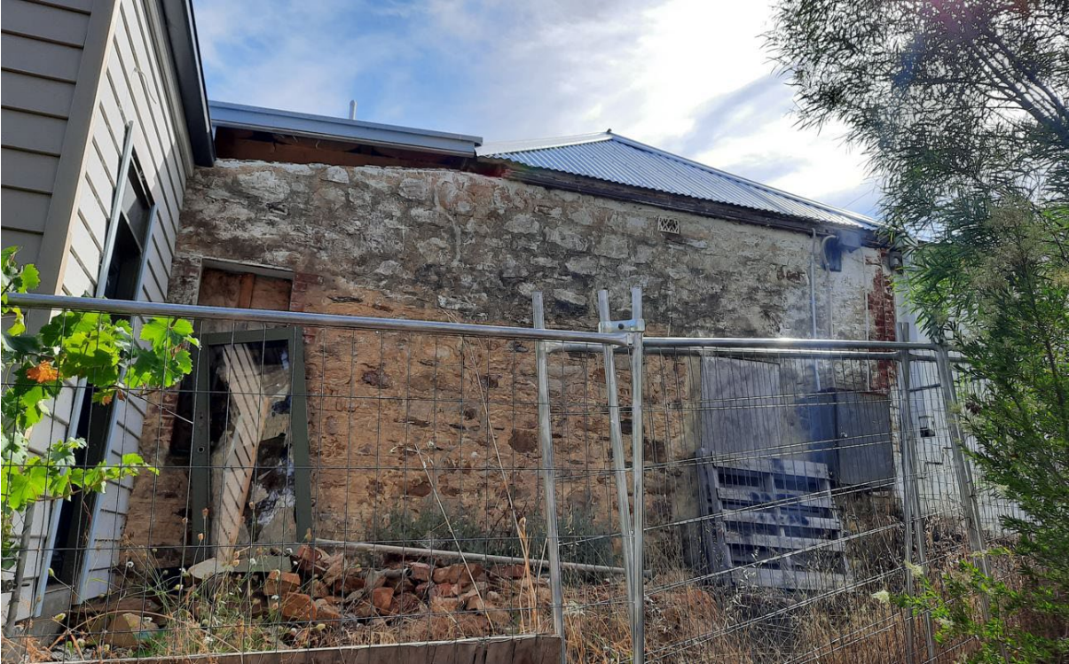
South elevation of c.1902 cottage, showing deteriorated fabric and current repairs (GGA, 2022)
