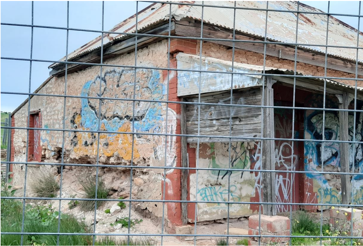
East elevation of former farmhouse, currently in dilapidated condition (GGA, 2021).
