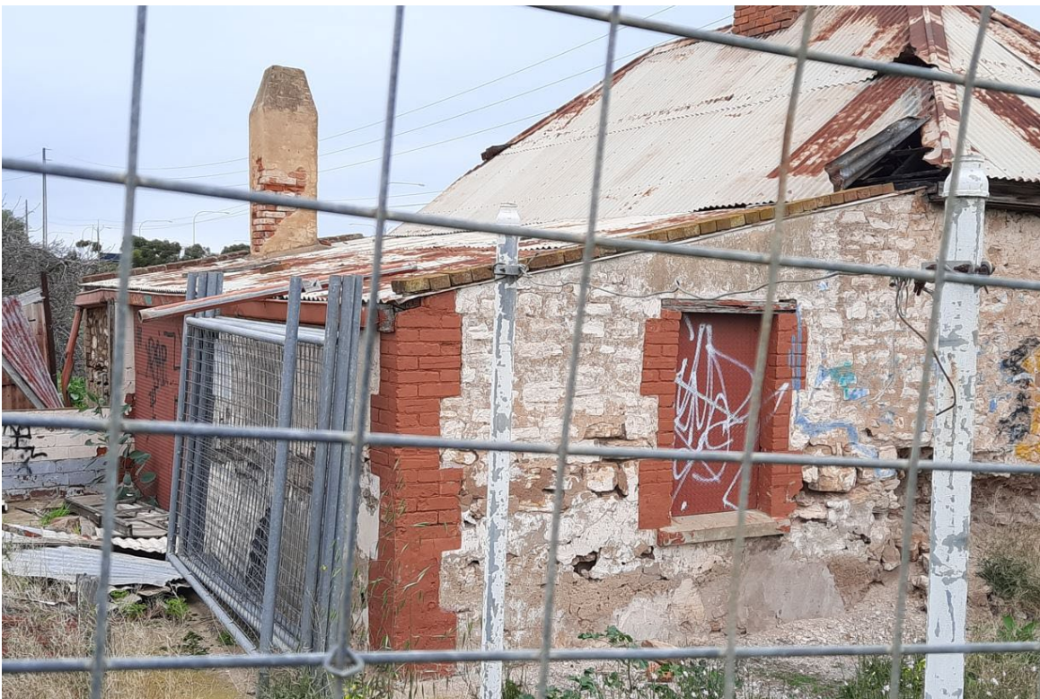
Southern lean-to additions to former farmhouse with various areas of external rendering, currently in dilapidated condition (GGA, 2021).
