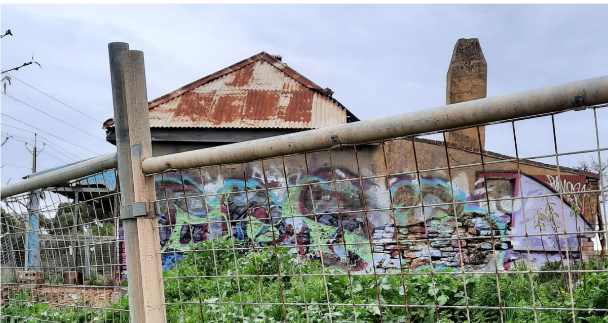
West elevation of former farmhouse, currently in dilapidated condition (GGA, 2021).
