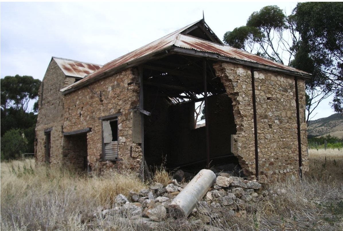
Dilapidated chaff mill in 2014 before commencement of reconstruction works (image courtesy of current owners).
