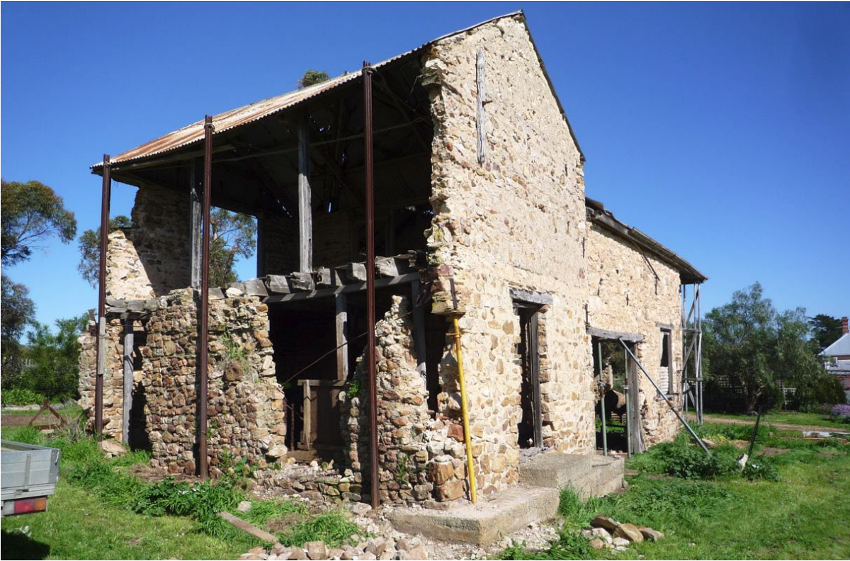
Dilapidated chaff mill in 2014 before commencement of reconstruction works (image provided courtesy of current owners).
