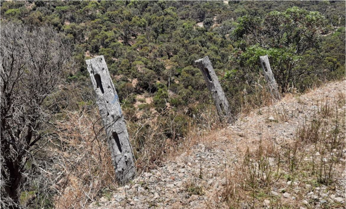
Examples of typical early timber fencing to Old Sellicks Hill Road, now in various states of decay (GGA, 2022).
