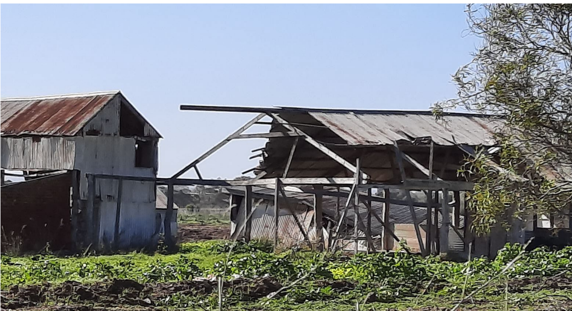
Barn/shed ruins now extensively dilapidated; note collapsed shed in background (GGA, 2021)
