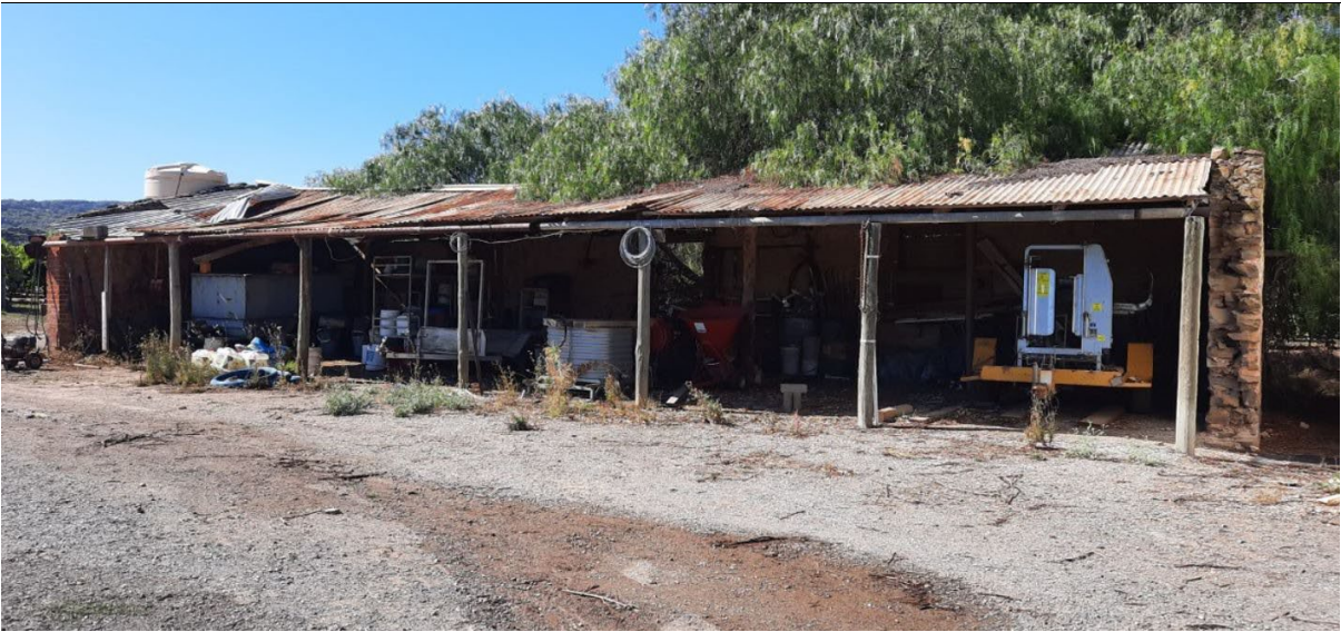
Current dilapidated appearance of the former coachhouse at 100 Delabole Road, Whites Valley, looking south (GGA, 2022).
