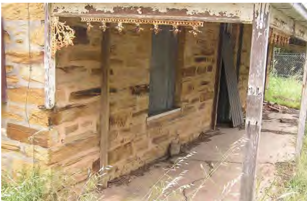
East elevation of former 'Rowlands' farmhouse, showing original masonry with later timber verandah with cast iron filigree brackets and friezes. (Andrew Stevens photographer).
