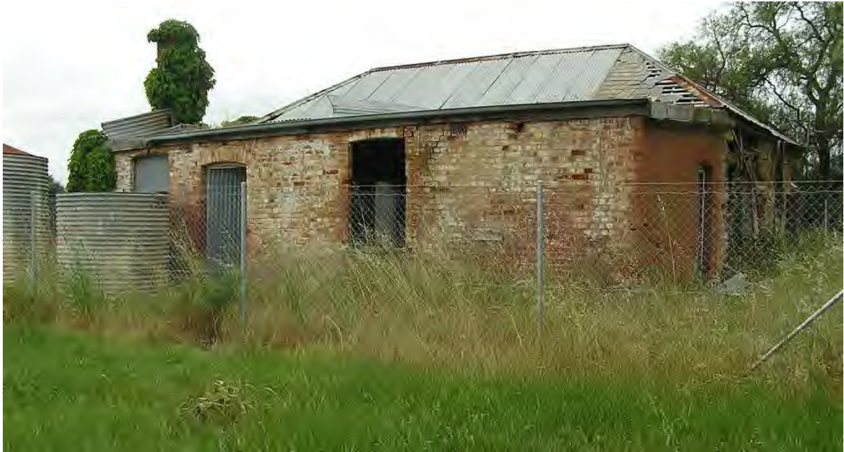
West elevation of former 'Rowlands' farmhouse, showing early 20 th century rear lean-to additions and 20 th century rainwater tanks (Andrew Stevens photographer).
