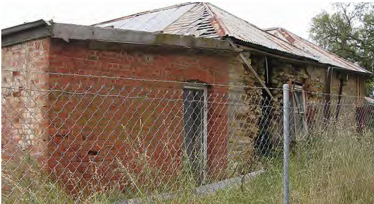
South elevation of former 'Rowlands' farmhouse, showing early 20 th century rear lean-to additions and slate roof tiling under later corrugated iron sheeting (Andrew Stevens photographer).
