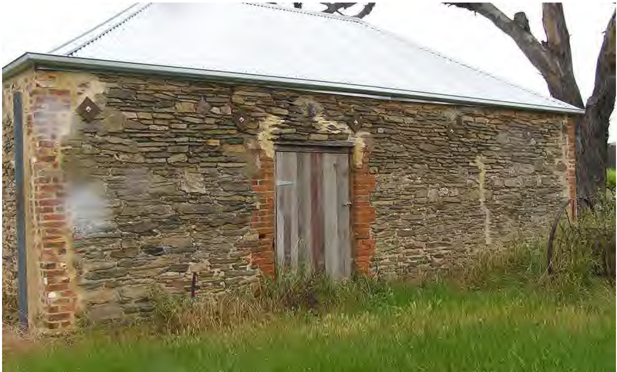
Masonry fabric of north wall of Outbuilding No.3, looking south (Andrew Stevens, photographer).
