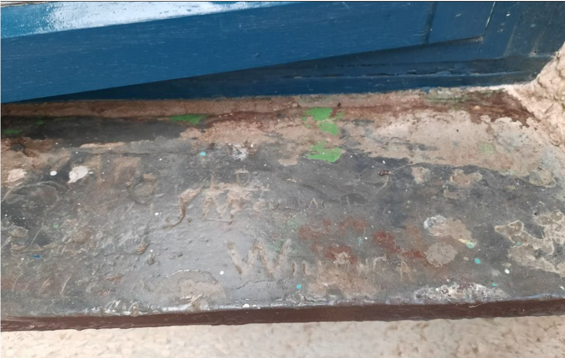
Early slate window sill with extensive inscriptions of former owners and residents of 24 St Peters Terrace, Willunga, dating back to the mid-19 th century (GGA, 2022)
